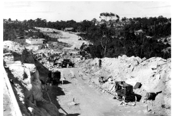
Building Stringybark Creek Bridge, Epping Road, (Main Road 373), circa 1939. (Courtesy of The State Library of New South Wales)
